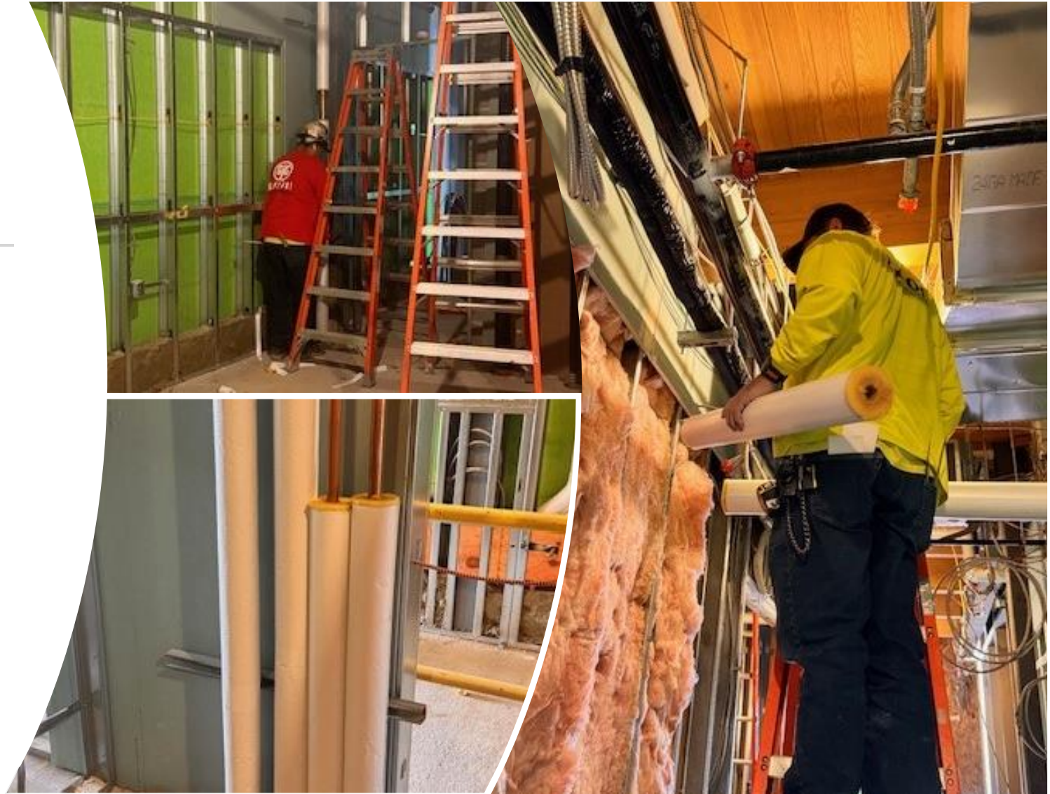
Copper water pipe insulation on second floor of the Utility Building
