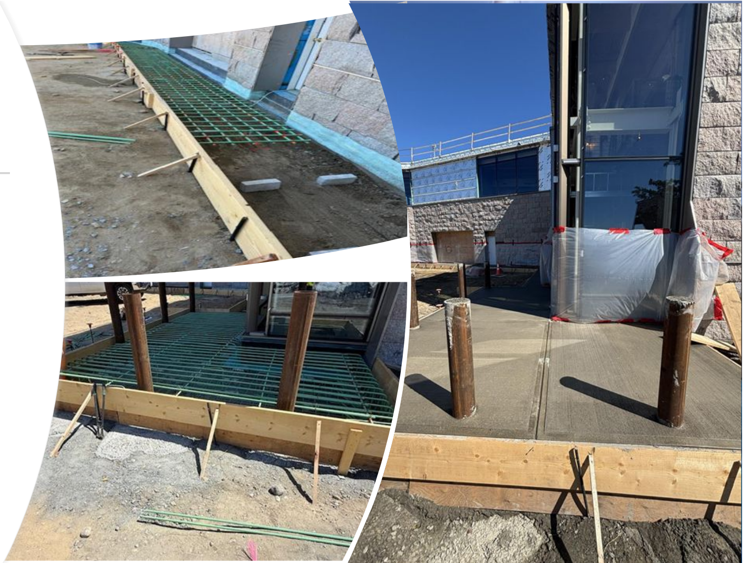
Parameter protection walkway at the North side of the Utility Building.
