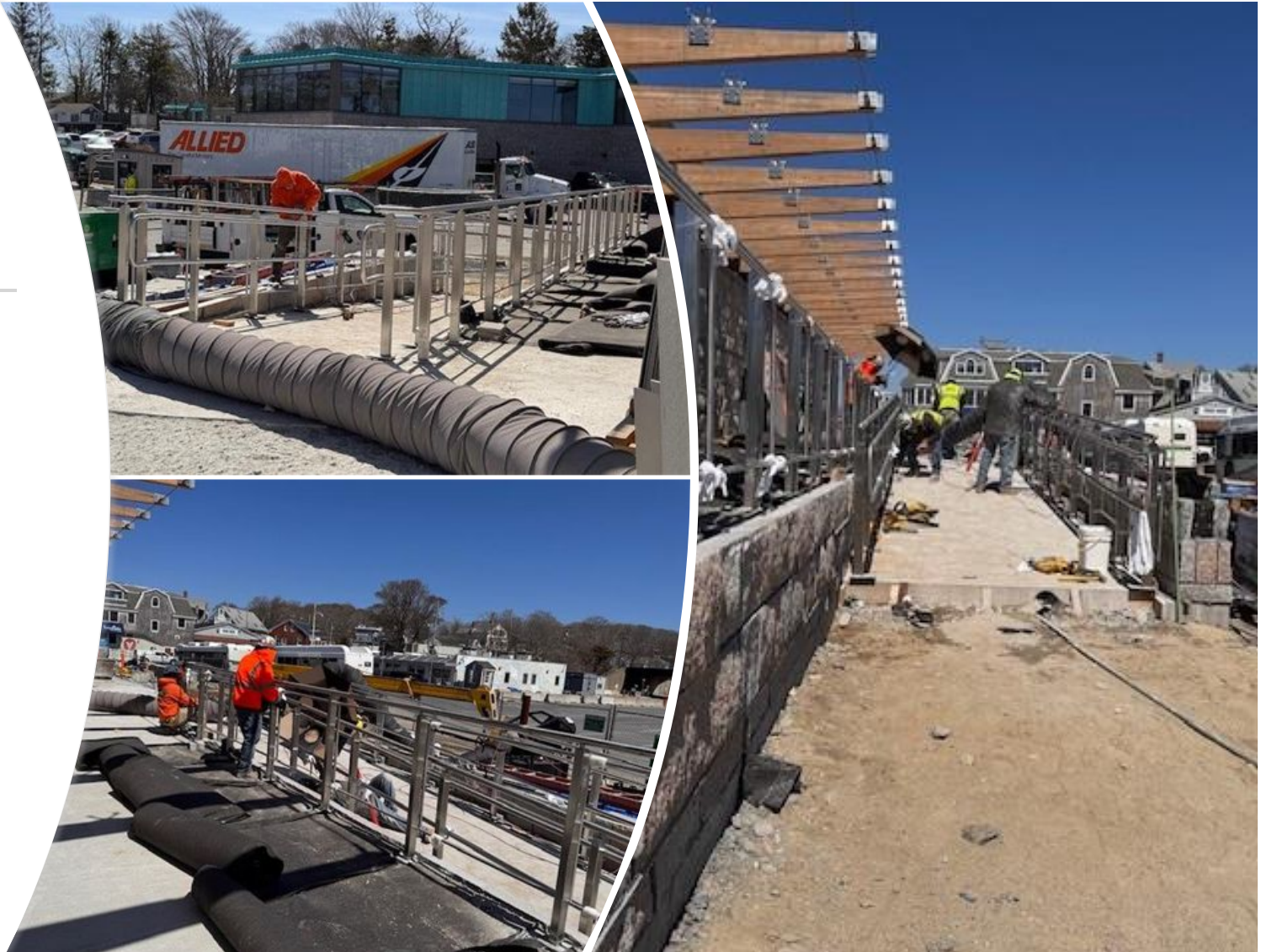
Railings are installed at the ramps and patio on the East side of the Terminal Building
