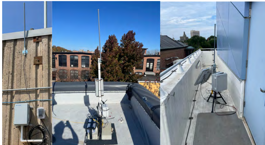
Figure 3: Example of gateway setups with hardwired power and internet (left), hardwired power and cellular internet (middle), solar power and cellular internet (right).
