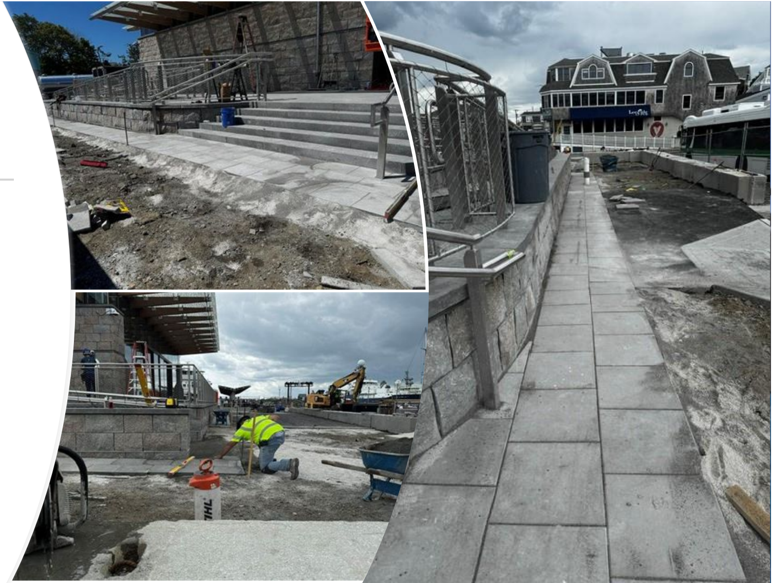
Pavers are installed along a future sidewalk area at the perimeter of the Terminal Building
