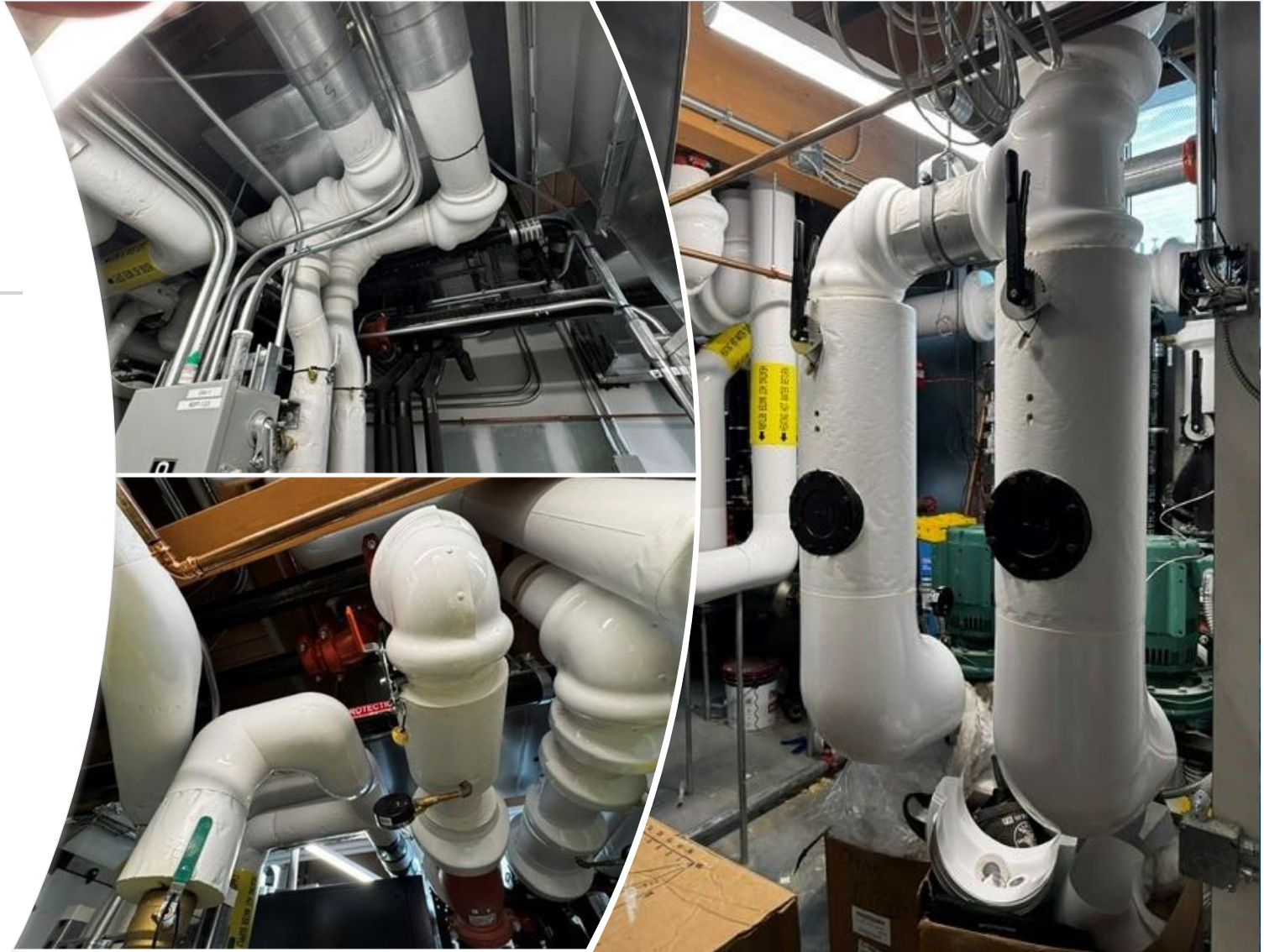
Copper and cast pipe is wrapped with pipe insulation throughout the Mechanical Room
